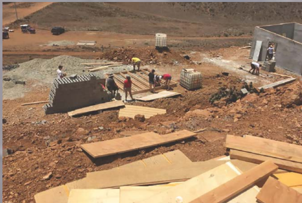
Construction in Hope Village is underway. These will be the homes of single women and their families who have been neglected and abused in the near future.
